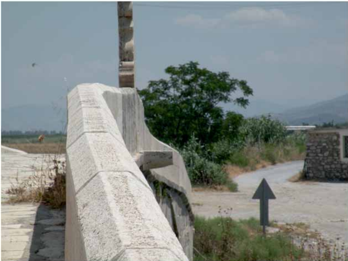
Figure 12. Deformed Ramazanpaşa Bridge over the Maiandros river (Photo by Ökmen Sümer)
